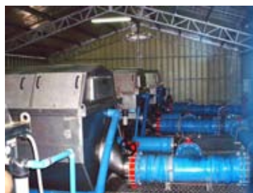
Inlet filtration to hatchery and on-growing facilities. Filters are tank versions, HDF1605-1H
